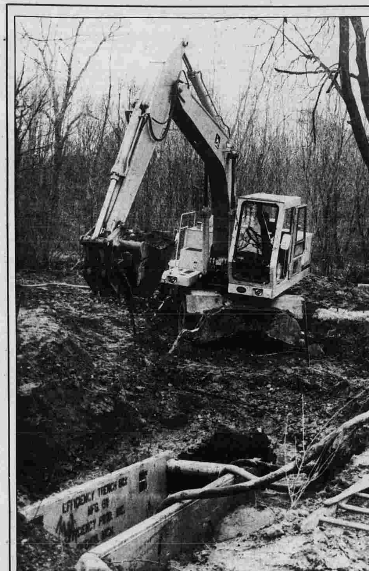
MAIN MATTER — An employee of the Manchester Water Department's Construction Division uses heavy equipment Monday to install a water main under Porter Brook behind the department's garage.
